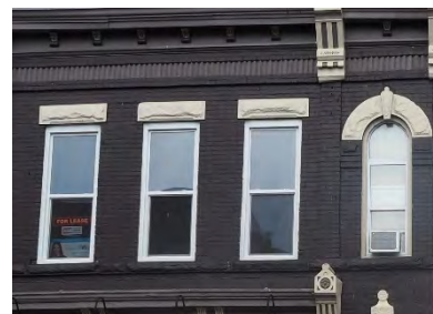
A large percentage of the brick surfaces in the HCD have been painted. Avoid painting masonry or using abrasive cleaning techniques.
