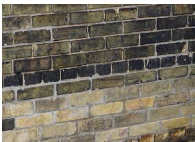
Colour difference due to accumulation of dirt on brick. Cleaning for aesthetics reasons may be considered.
