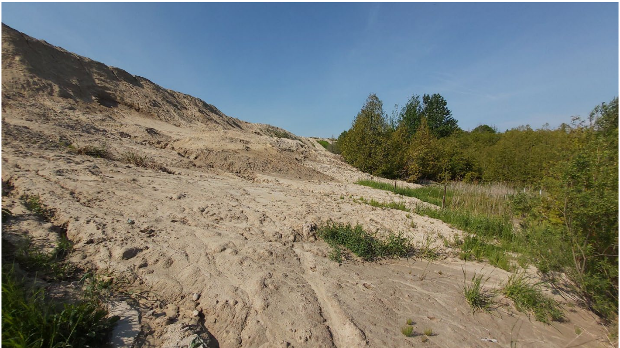
Photo 27– Sloughed stockpile near Slope Incliner SI-03, looking south (May 31, 2022)
