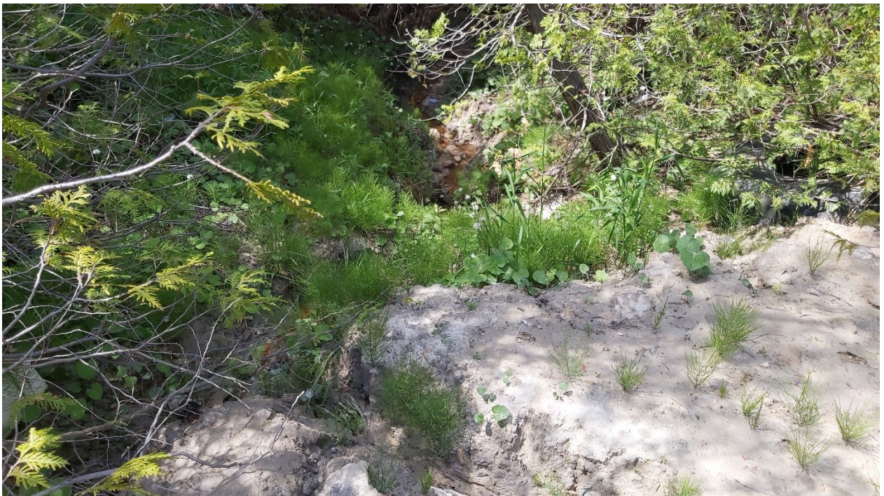
Photo 30 – Sloughed silty soil in front of New Survey Pin SP-7, looking west (May 31, 2022).
