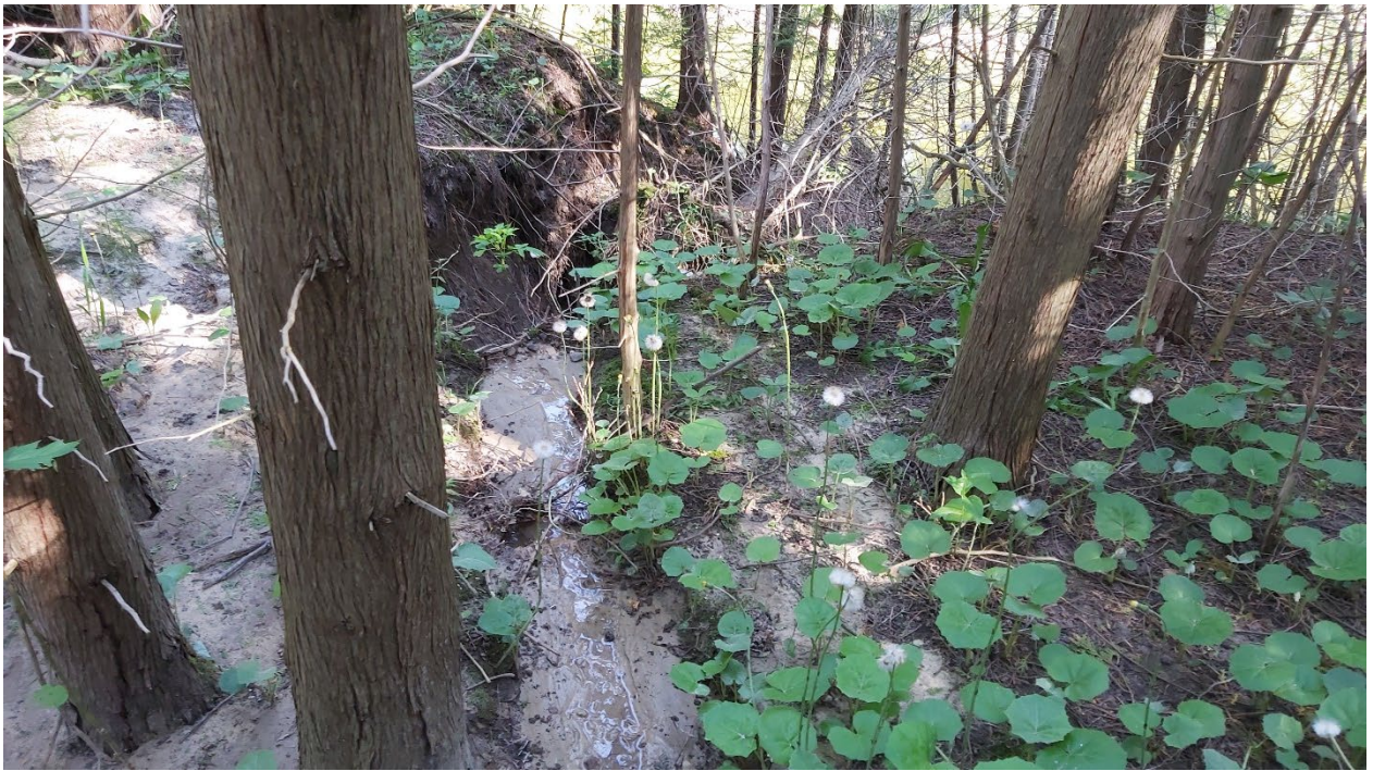
Photo 15 – Loss of tree roots and erosion gullies north of Survey Pin SP-5, looking southwest (May 31, 2022)
