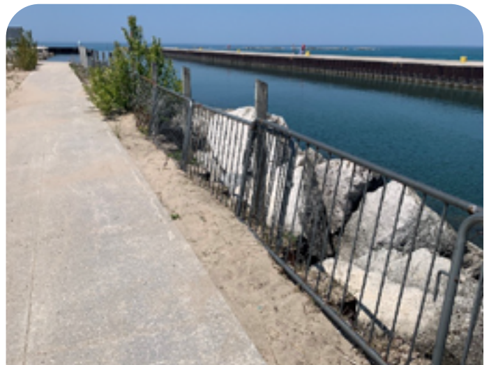
North side of South Pier. Fencing poorly situated for the purpose of keeping patrons from entering the path of vessels maneuvering the harbour mouth.
