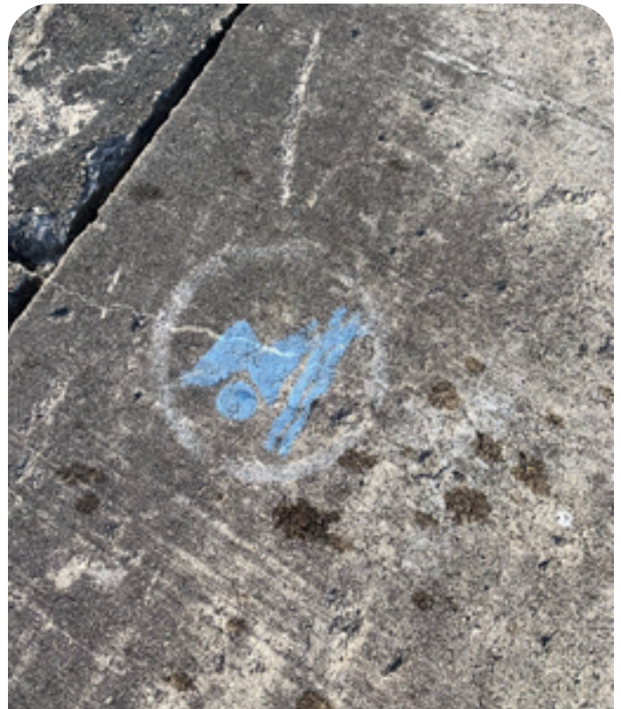
Existing painted stencil on Kincardine Pier to depict No Swimming.
