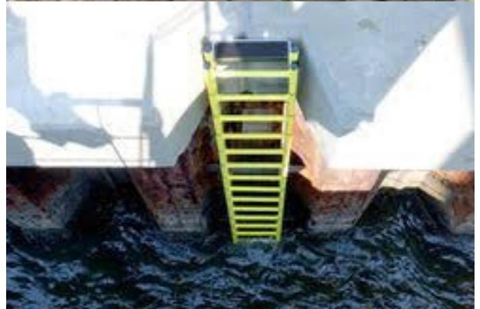
Example of new ladder system.
