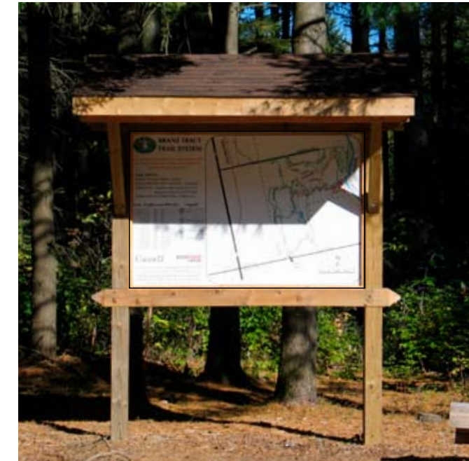
Structure for kiosks constructed to match existing Brant Tract Trail System kiosk.
