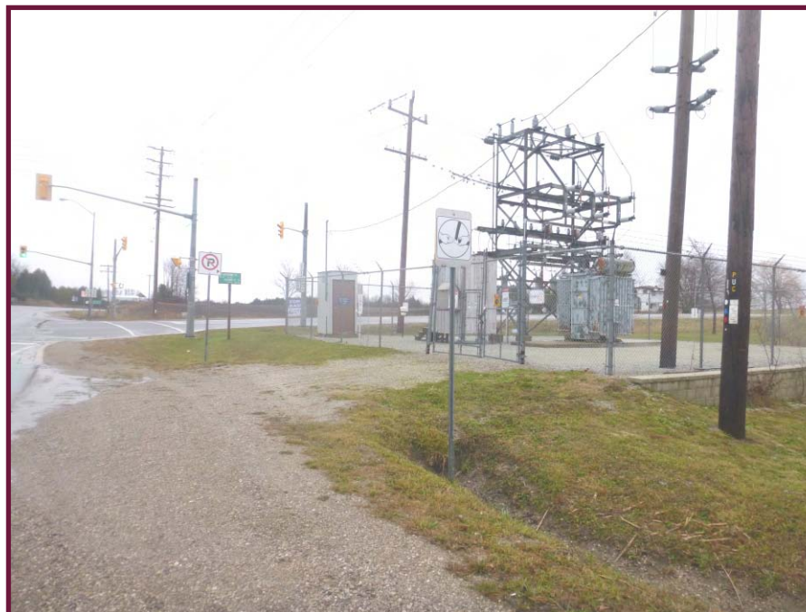
Image 5: Transformer Station in Northwest Corner of Study Area (looking northeast)
